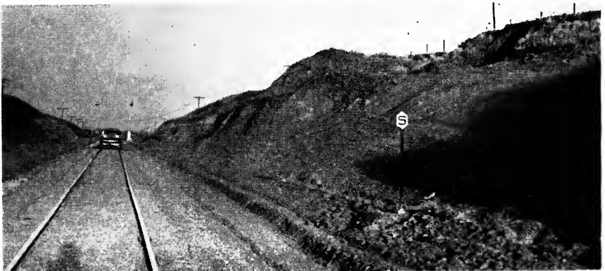
Fig. 2—Pottsville-Sadler revision, slides in cut slopes, 1948.
